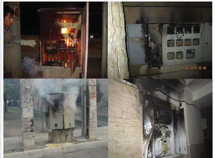
Figure 1: Damage caused by rising temperature in electrical panels.
